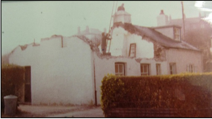
LEFT This is a 1979 photograph when the old roof was taken off. There were two rear downstairs windows at that time, and on the gable end at the top can be seen the shapes of the small windows either side of the old fireplace in the upper room.
