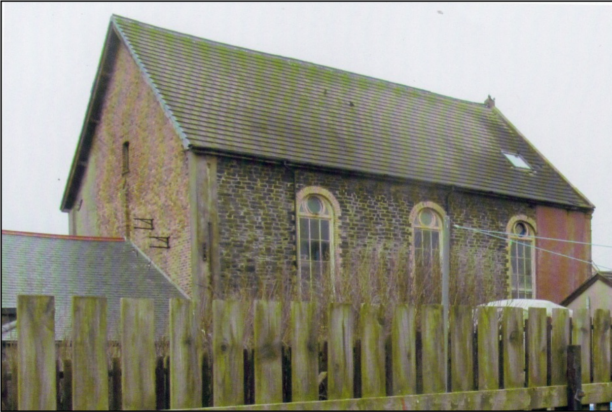
ABOVE This is the north wall of the building seen from the garden of Pomona. The walling of this main section of the building is dressed rubble stone. The windows are edged with yellow sandstone.
