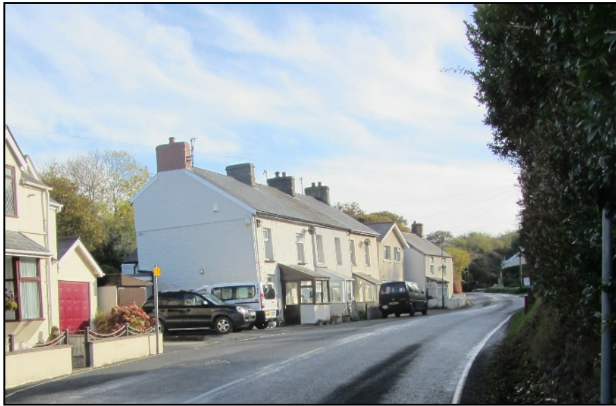
ABOVE In 2015 the terrace was leaning backwards as a result of drainage operations on the marsh at the rear.
