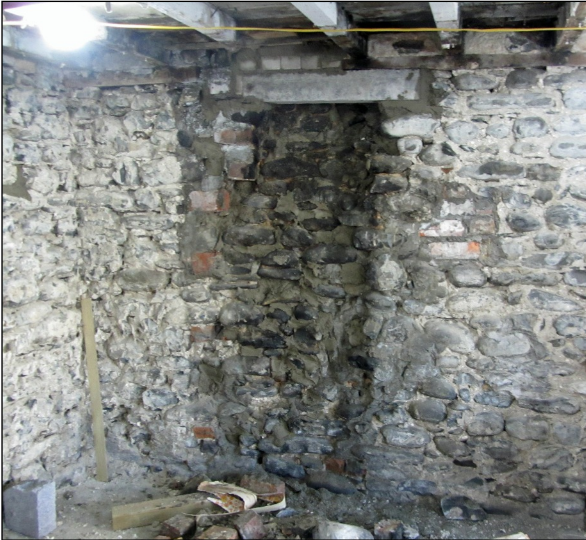
LEFT The north and rear wall of The Art Shop was stone with rounded stones from the beach and its chimney in the centre of the picture was also stone.
