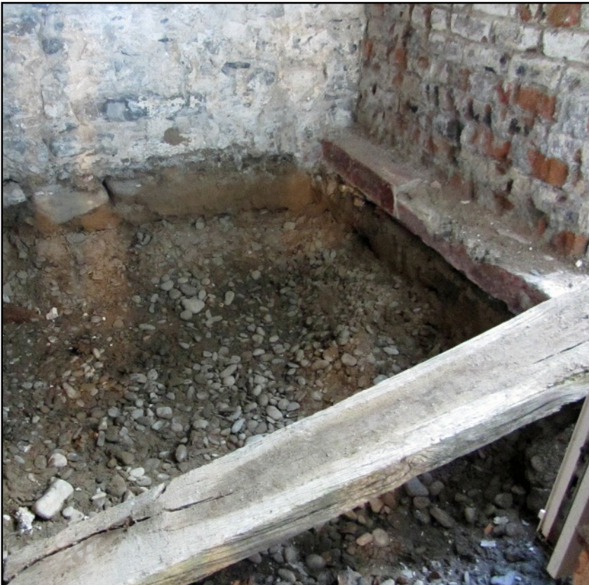
LEFT Below the floors was sand and gravel and the sill to support floorboards can be seen on the right. This left an air space to prevent damp.
