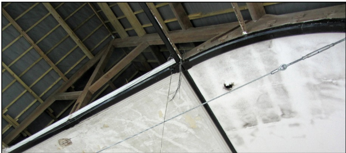
ABOVE The metal tie is a recent safety measure to stabilize the building.
