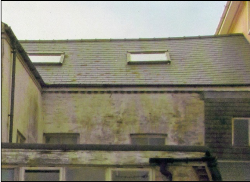
LEFT Beneath the rendering at the back of the building are traces of a stone wall beneath. Under the eaves is a pattern usually caused by protruding wooden beams ends or bricks.
