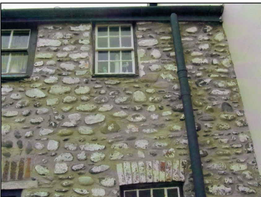
LEFT Dark red bricks with the remains of whitewash left on them make a shallow arch above the right hand ground floor window.
