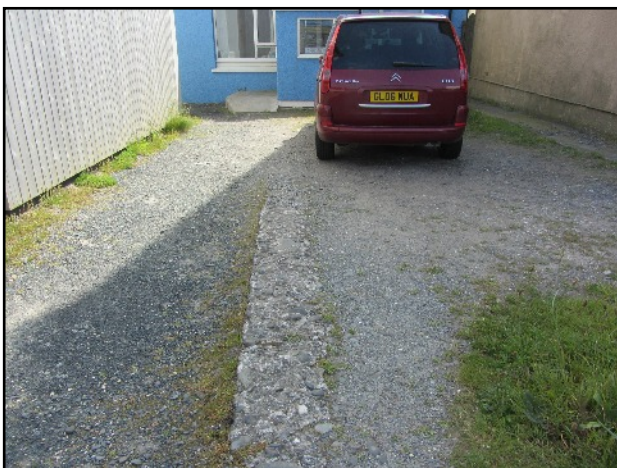
ABOVE A section of old stone wall remains leading from the north gable end of the cottage. This is topped with brick shaped stones.
