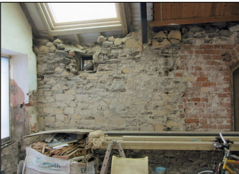
LEFT Some of the old stonework survives on the north wall at the west end. There are some sizeable and good quality stones. The roof light is part of the re-building.
