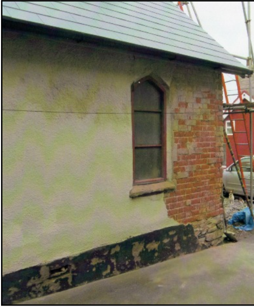
LEFT This is part of the south wall showing it has a footing of stone and some of the brick walling.
