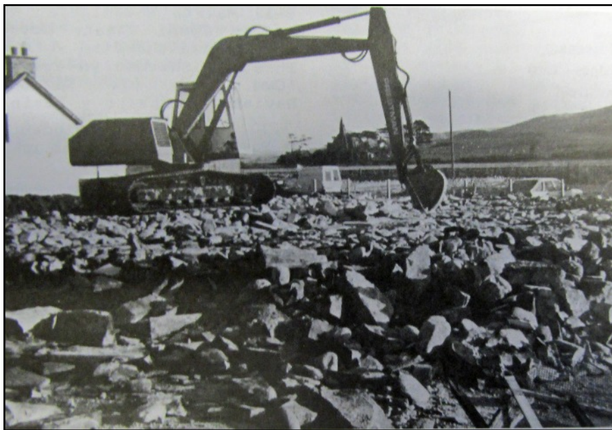
ABOVE The demolition of the school, Y Tincer February 1995 (Photo by courtesy of Y Tincer).
