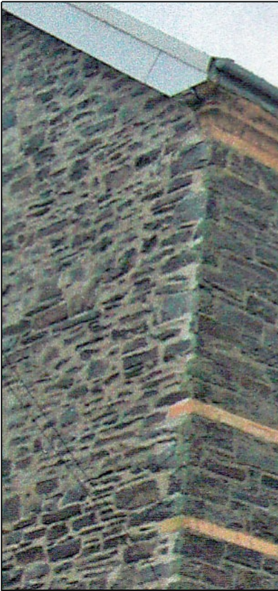
LEFT The random rubble stone of the north wall of London House.
