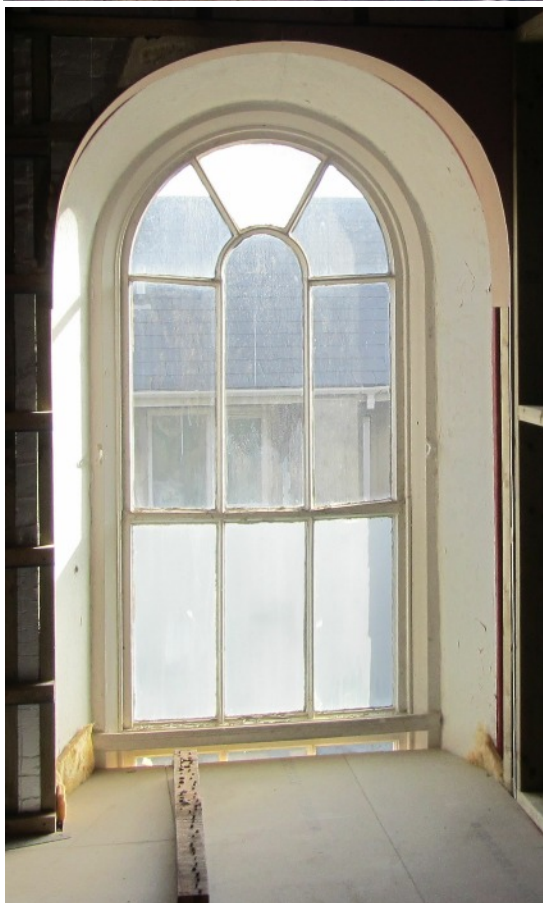
One of the classical style windows taken during re-building work in February 2016.
