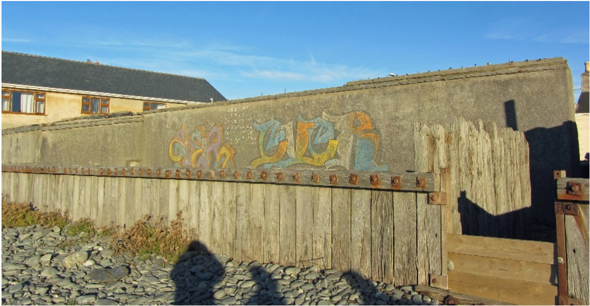
This is the rear of the Lerry Garage Site in 2016. The rear wall was probably left as a defence against the sea during bad storms. On the right is the passage from the High Street to the sea.
