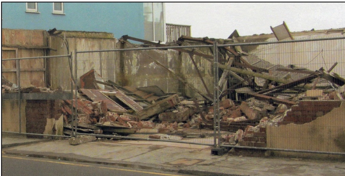
ABOVE Spring 2014 during the demolition of the building. The colour of its red brick wall and some rendering can be seen in the foreground on the right.
