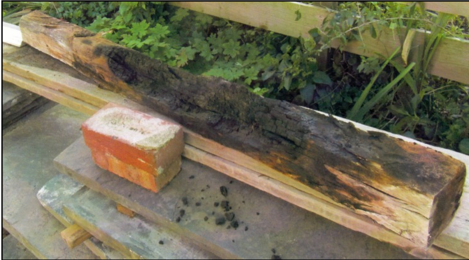
LEFT The original beam above the fireplace was badly burnt in places.
