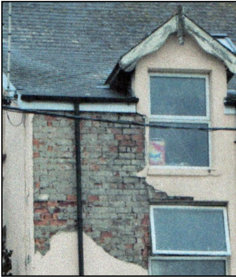
LEFT Most of the walls are hidden under the rendering, but this area on the extension has grey and pink coloured bricks.
