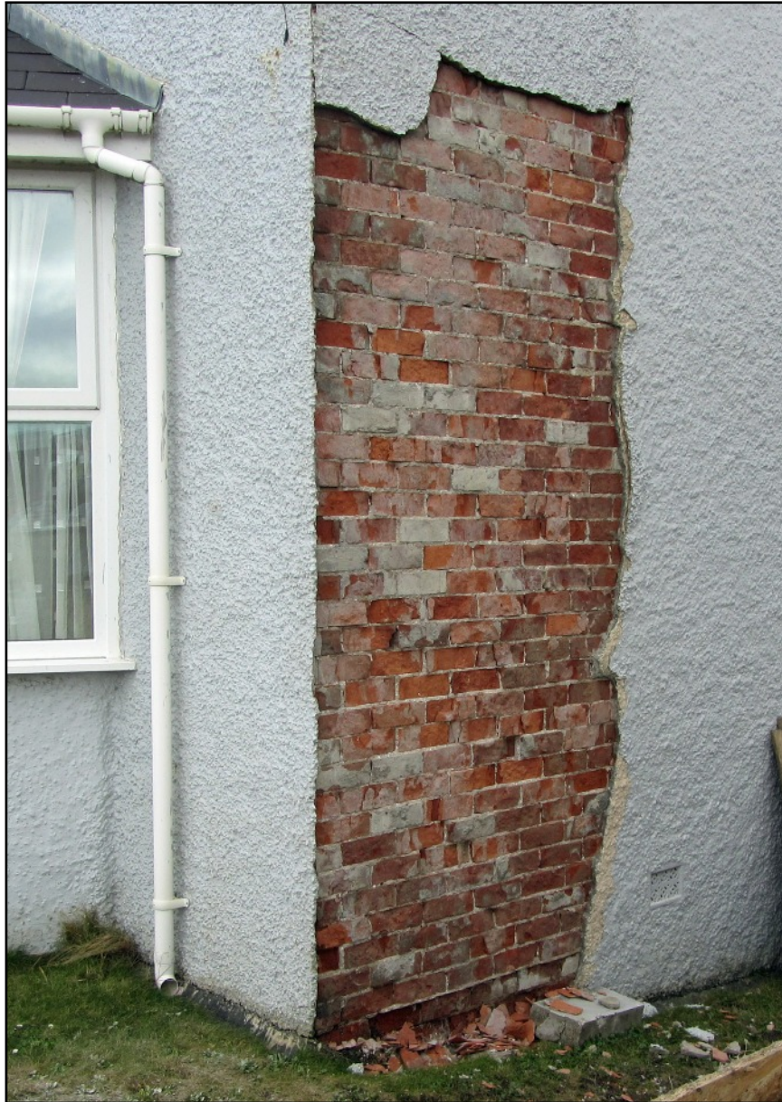
ABOVE During work to build an extension on the east side rear of the house in 2019 this area of wall was cleared of rendering and it was possible to see the brickwork of the walls.
