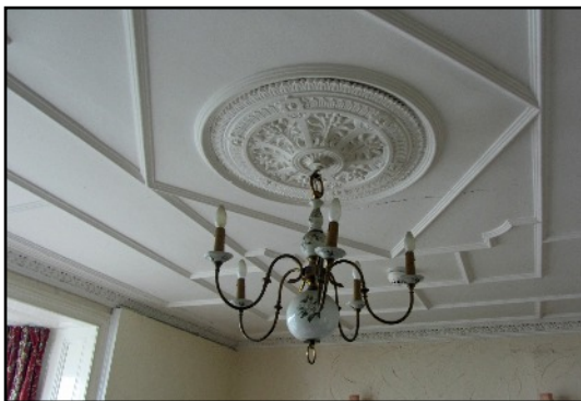
ABOVE The ceiling plasterwork of the front ground floor room.
