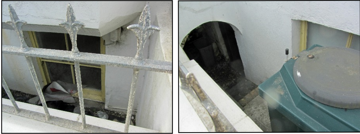
ABOVE The basement window on the south of the front door, and the entrance to the basement and its other window on the other side. The sash windows match those on the rest of the front of the house.
