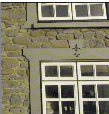
LEFT Smooth plaster shapes edge the windows, with a fleur de lis decoration on a keystone at the top of the lower windows.
