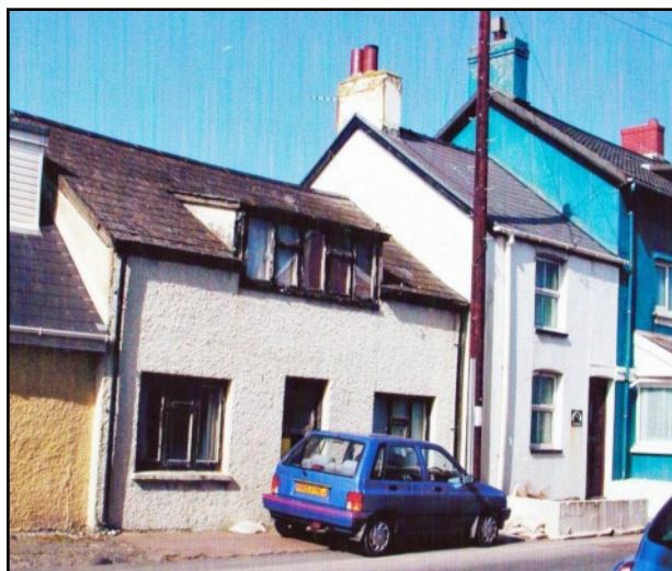
LEFT Cartref in 2009 showing how narrow the building is between Leander on the left and Glasfryn on the right.
