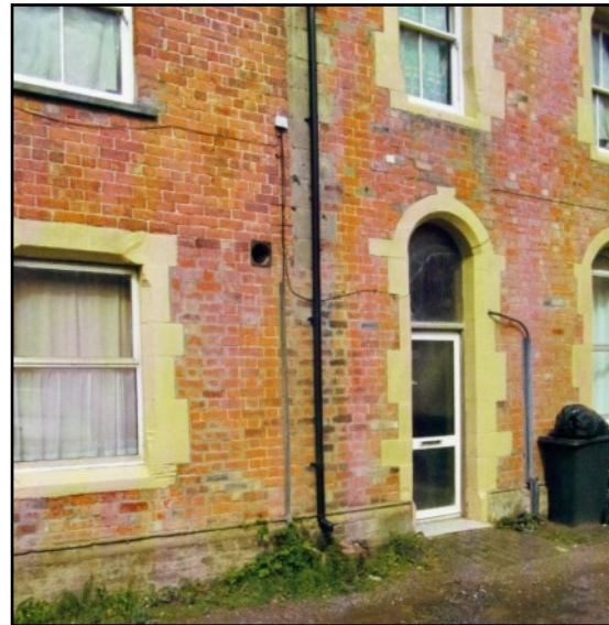
ABOVE The east side of Rutland House (Number 1) has been cleaned, showing the colour of the bricks and the sandstone dressings.
