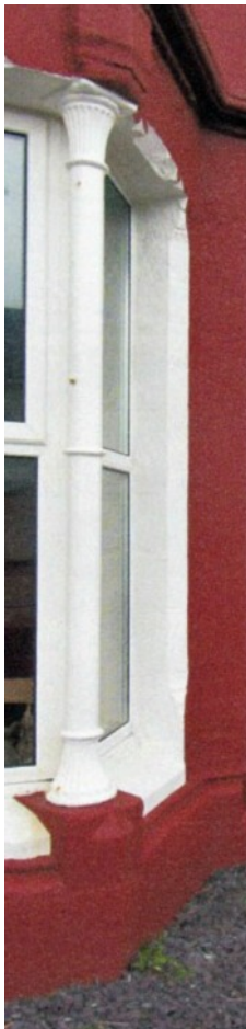
LEFT A column on Number 4. These were in the Gothic Style, and their central ring matches the centre of the sash windows. They had to be made in two sizes as the ground floor windows were taller.
