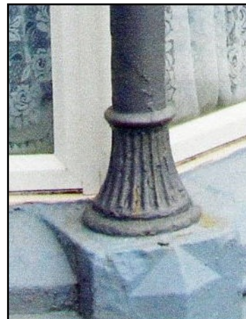
LEFT The carved shapes of the sandstone dressings have survived on Number 10. The columns had a special top and base, and the chamfers above the window and door have decorative ends. However if allowed to rust the iron columns make unpleasant stains on the rendering. The front door is modern
