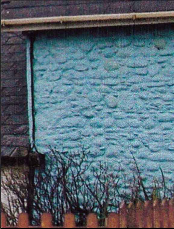
LEFT The north stone wall has a large proportion of rounded stones from the beach of all sizes.
