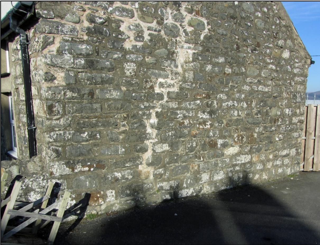
ABOVE The rubble stone of this cottage is interesting. Some stones are rounded from the beach, and others are large, and coursed. This is the south gable end.
