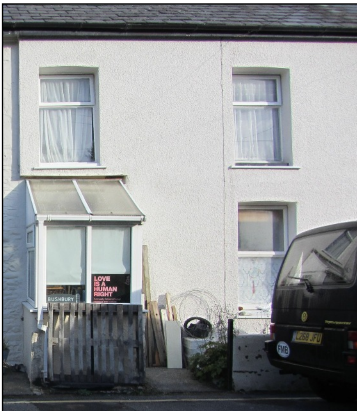
ABOVE The front of Bushbury in 2015. It is notable for its very smooth rendering.
