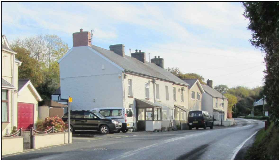
ABOVE Today (2015) the terrace is leaning backwards owing to subsidence from drainage operations. This did not crack the shell of the house though the floors can seem uneven.
