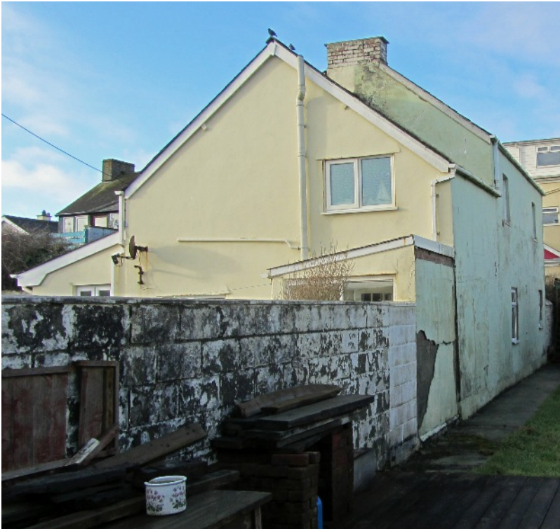
LEFT The rear of the house in 2018. There is a further small extension against the boundary.
