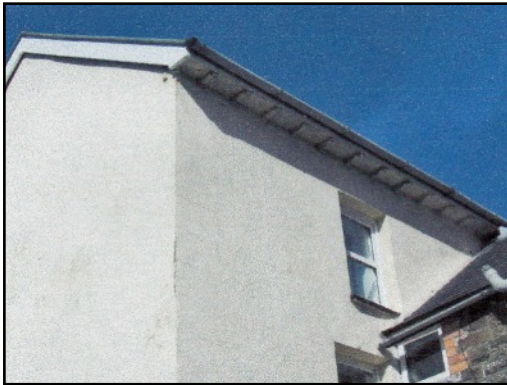
LEFT The overhanging roof at the rear has a pattern of beam ends under the eaves.
